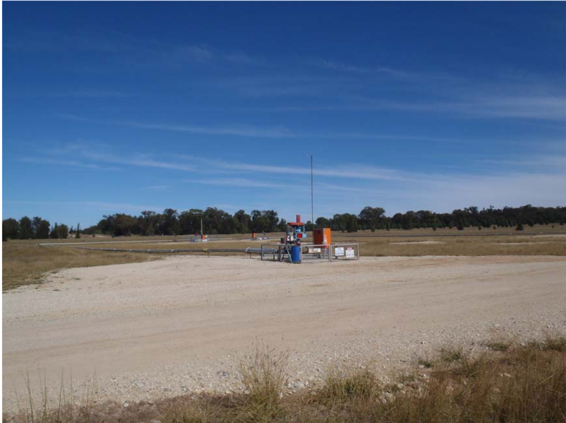
Plate 1 - Gas Drainage Infrastructure
