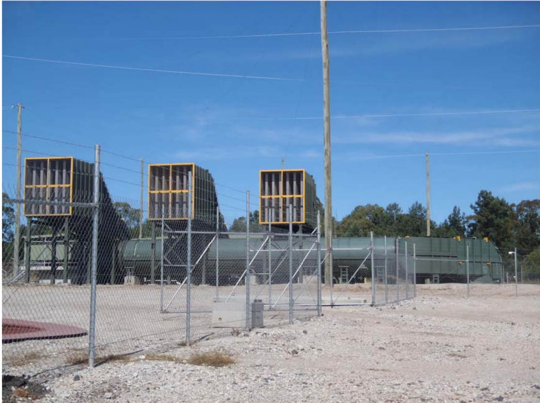
Plate 3 - West Mains Ventilation Fans
