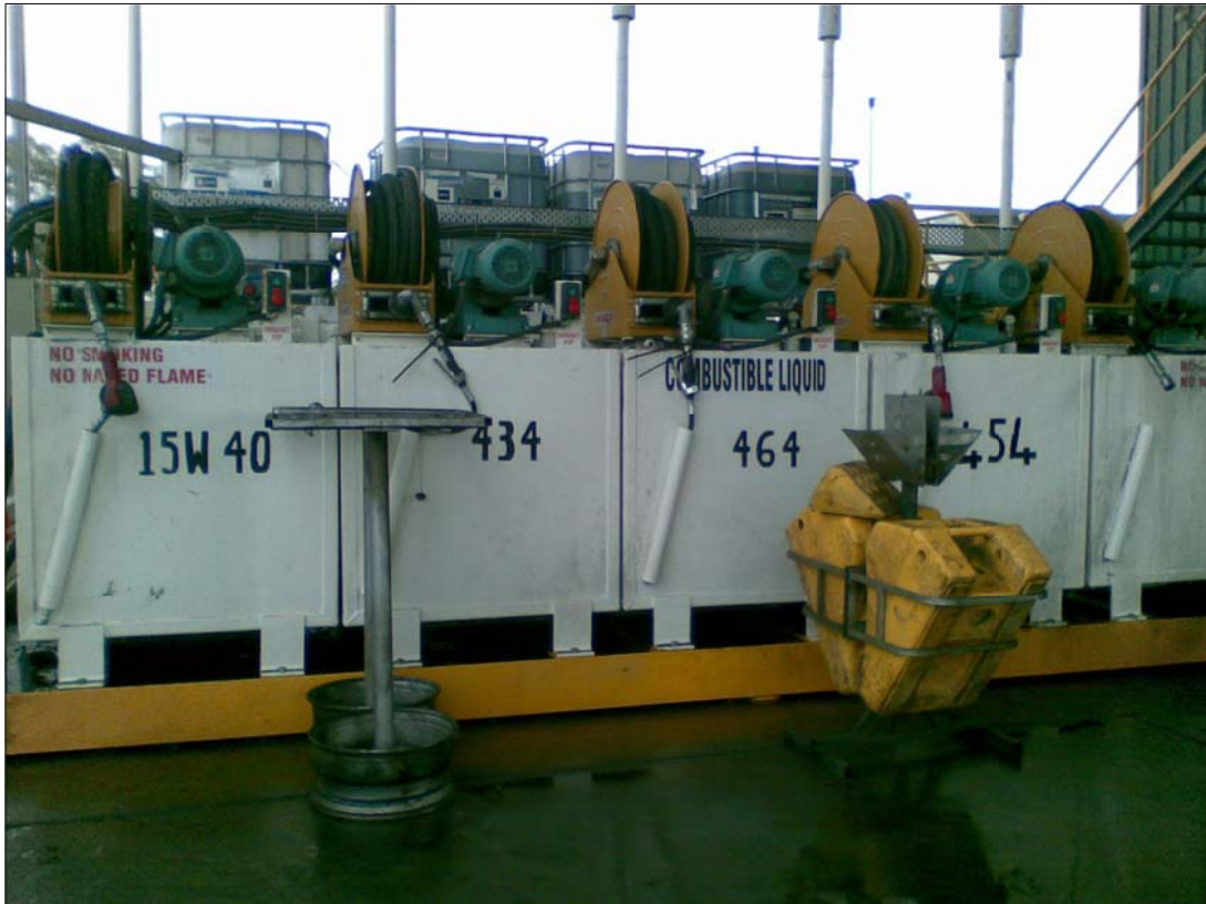
PLATE 5 Hydrocarbon storage at the workshop
